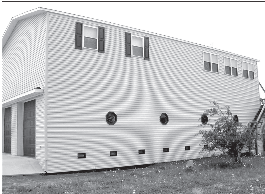
Figure 7. Manufactured home installed above a full-height framed garage (note elevation of driveway slab on left; the openings are within 1 foot of interior grade of the slab)
