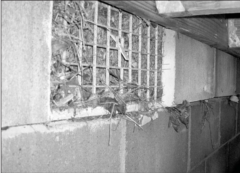
Figure 15. Typical air vent clogged by flood debris
