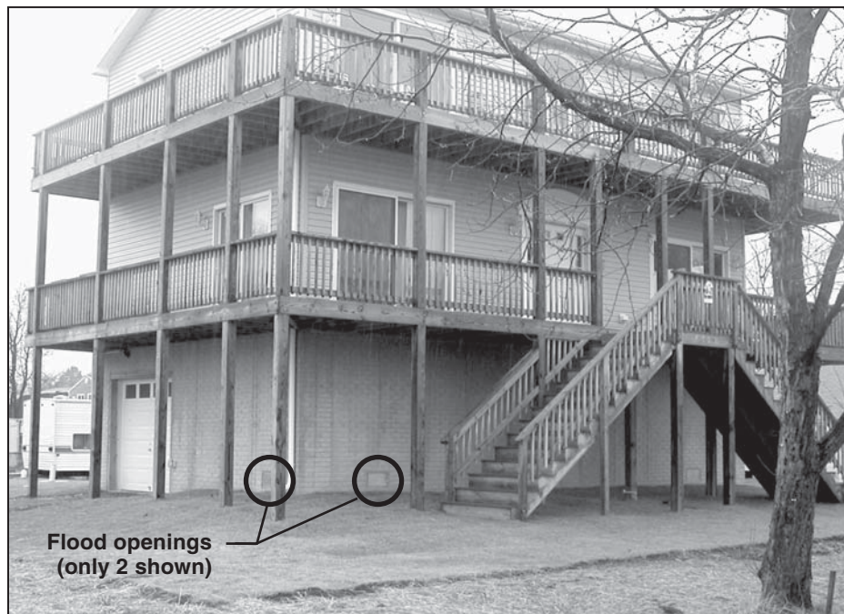
Figure 3. Full-height solid perimeter walls surrounding garage and storage area (only two openings visible)
